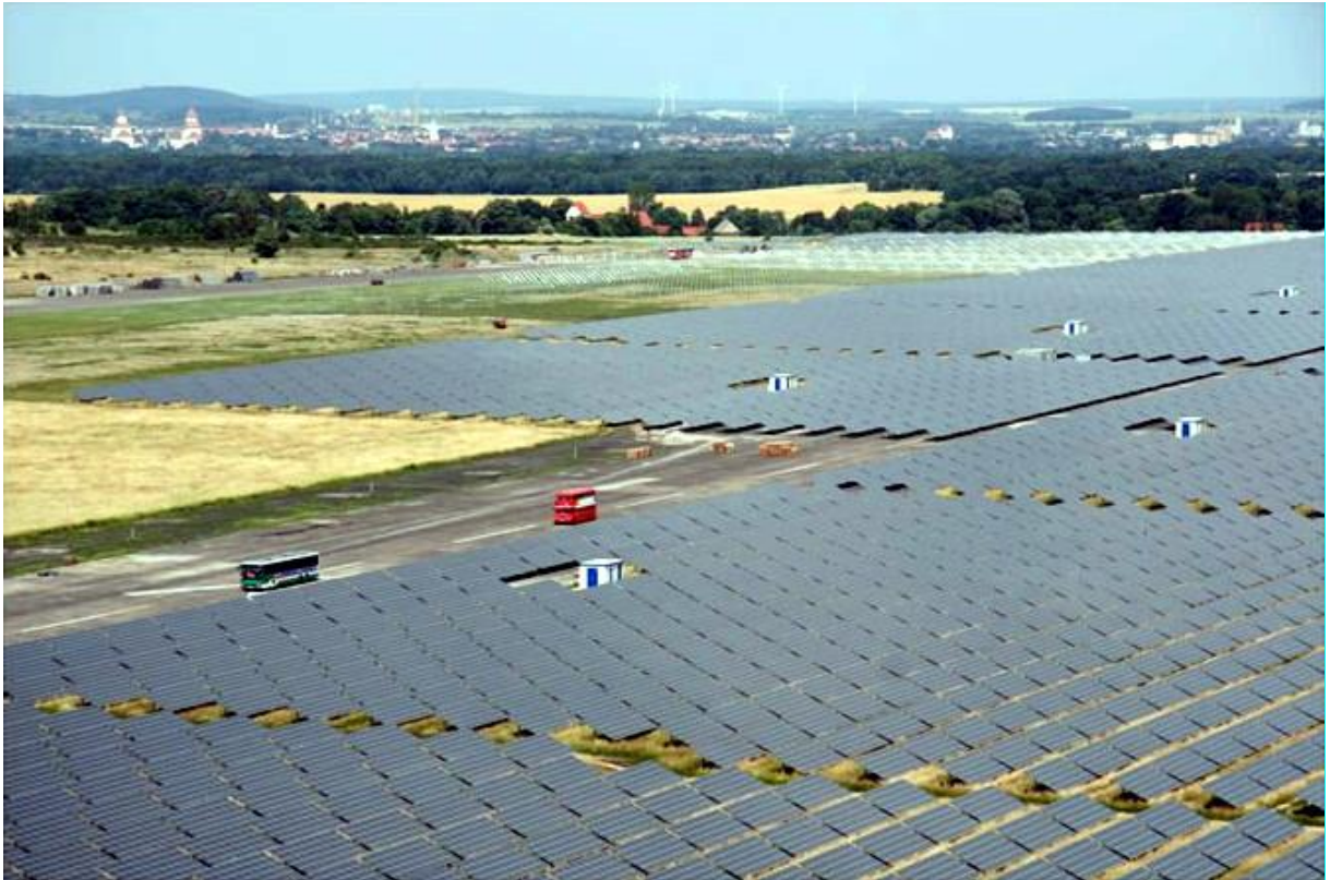
Figure 3 Free-field solar park (photovoltaic power plant) (Source: By JUWI Group - Photo courtesy of JUWI Group, CC BY-SA 3.0, https://commons.wikimedia.org/w/index.php?curid=4957243 )
